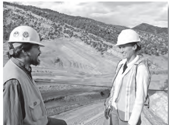
Standing on the south end of the future dam embankment, Barry Longwell, Animas-La Plata deputy construction engineer, explains Ridges Basin Dam construction operations to Karla Brown, CFWE executive director.
